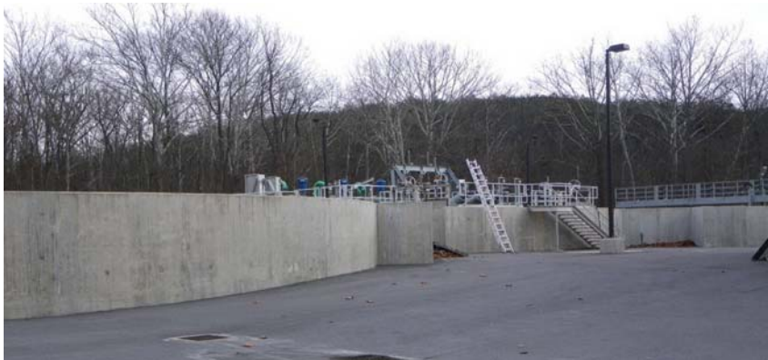
Figure26: Treatment basins at WSPSD wastewater treatment plant
